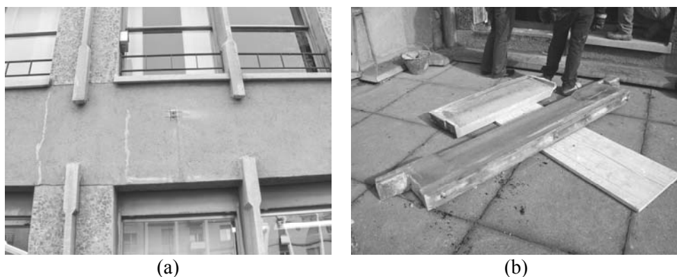
Figure 14 - Details of the small pilasters (a); and a small pilaster after being removed (b).
