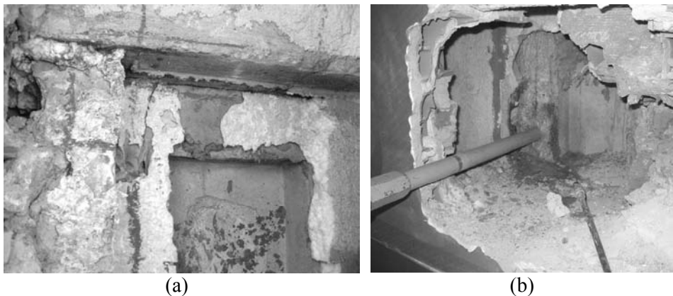
Figure 4 – Inspecting anchor rebars of precast elements with a pachometer (a); and a driller (b).
