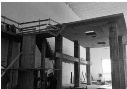
Figure 1 - View of the slab and of the columns (by courtesy of the firm “Milano Depur”, Nosedo Waste-Water Treatment Plant, Milan, Italy).
