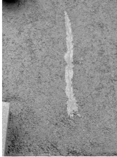
Figure 7 - Reopening of a repaired crack.
